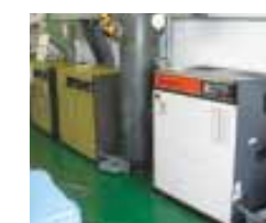
Auto-controlled compressors at Ono Works
